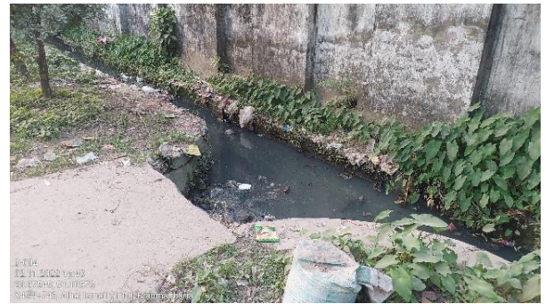
Drain-004, Brahmanbaria Paurashava
