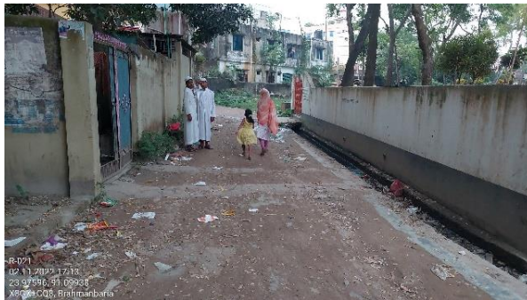
Drain-013, Brahmanbaria Paurashava
